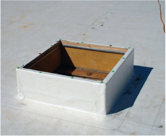
Flashing on an open top curb
