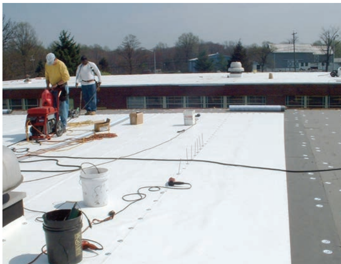
Mechanically fastened Flex TPO membrane
