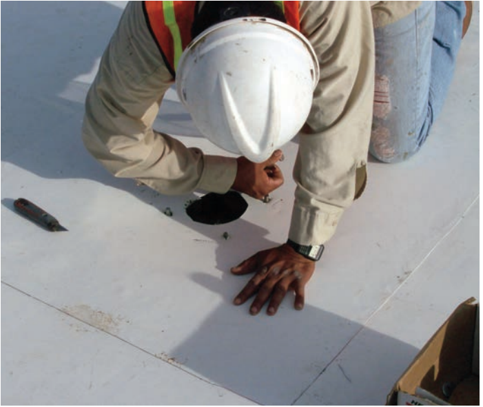
Installing a Flex TPO Flashing target sheet over the field sheet drain opening
